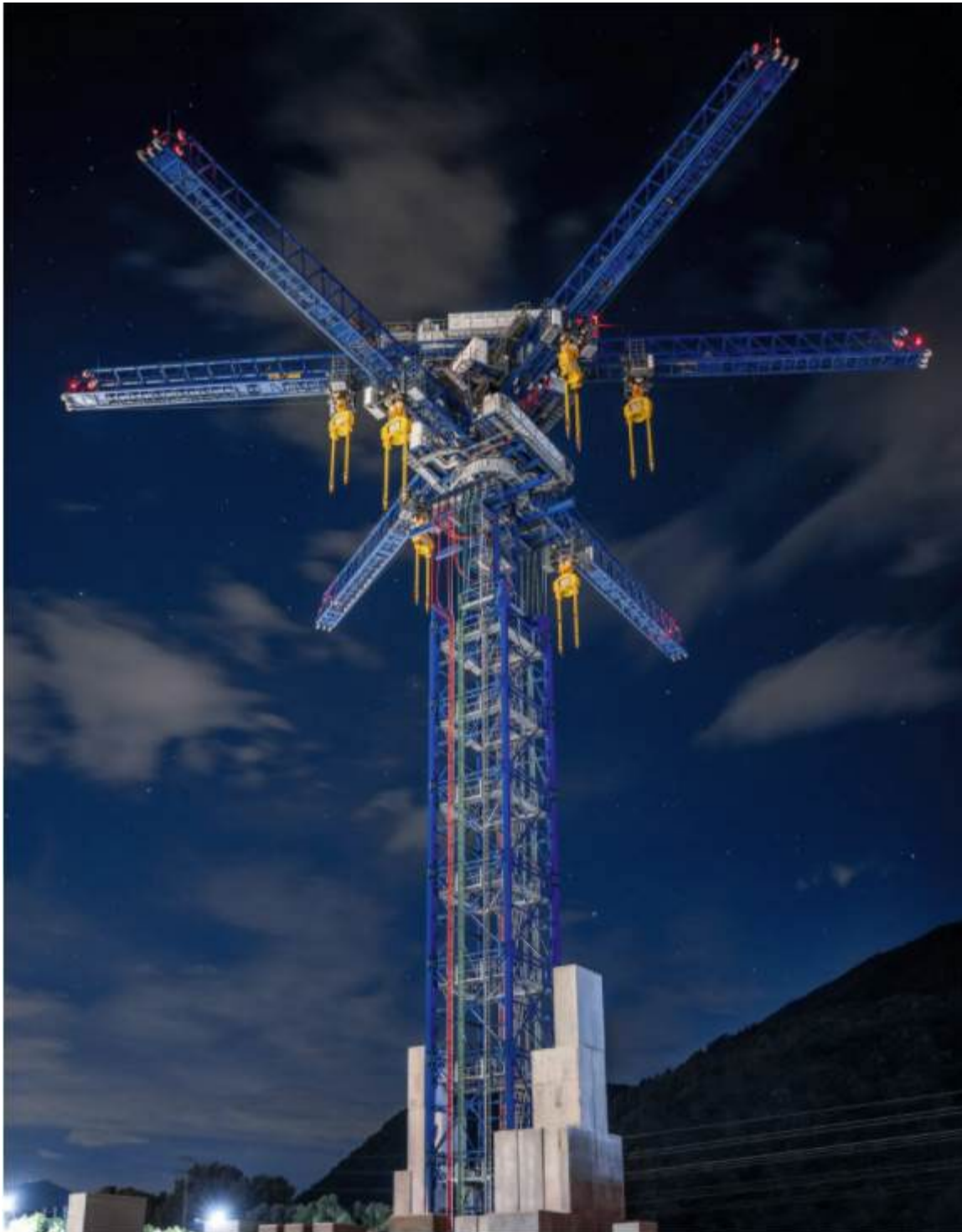
Energy Vault's 75-meter-tall Commercial Demonstration Unit at night, in Arbedo-Castione, Switzerland. PHOTOGRAPH: GIOVANNI FRONDONI
